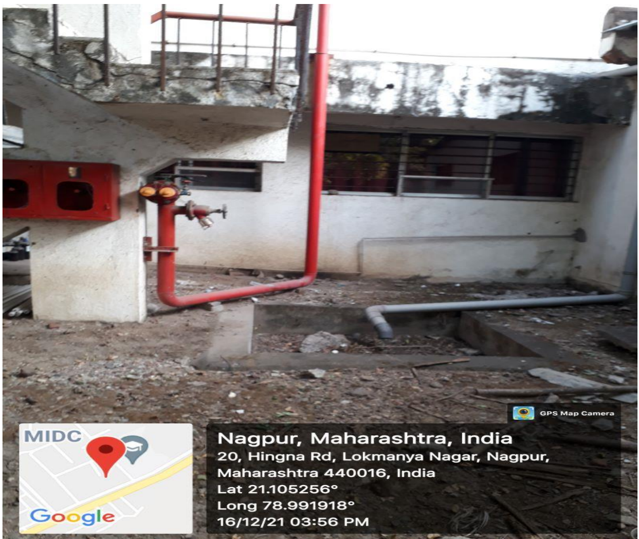
Rain water harvesting system
